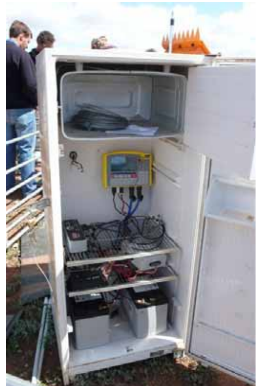
Remote weighing equipment housed in an old fridge
